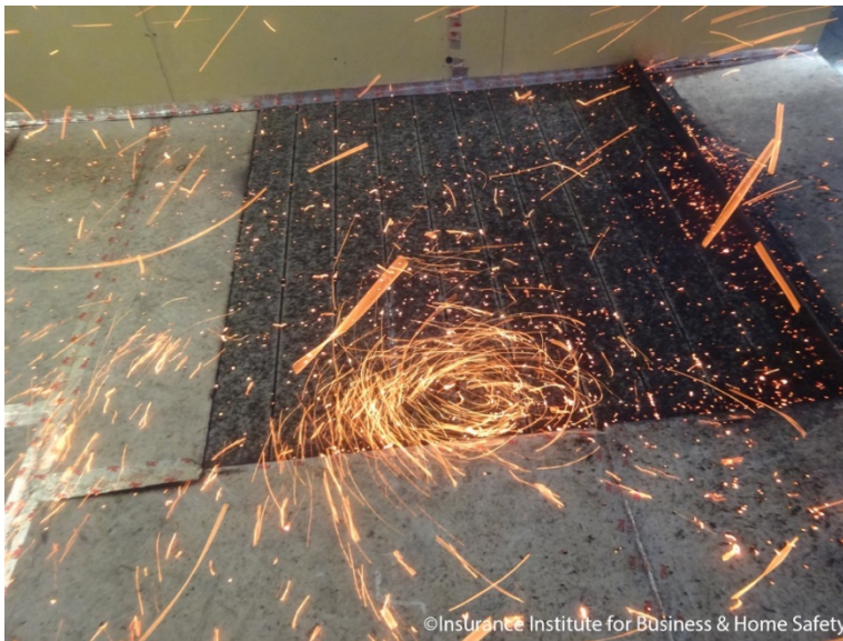
Figure 16. Ember accumulation areas on deck.
