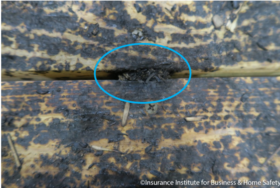
Figure 17. Ember accumulation in gap between deck board above a support joist.
