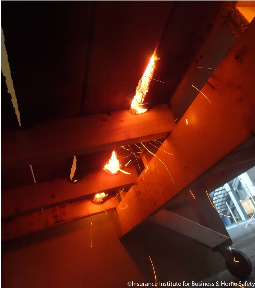
Figure 14. View of underdeck area. Flaming transitioned back to glowing/smoldering when the gap between deck boards and joists reached a point where flaming could not be sustained by radiant heat transfer.
