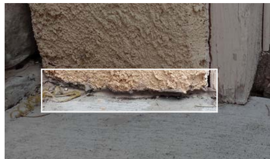
Figure 21. Gap between noncombustible siding and ground where debris and embers can accumulate.
