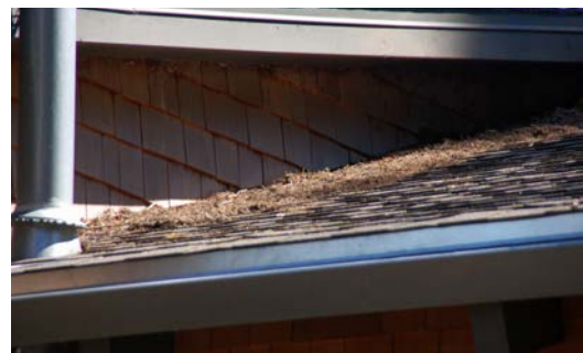
Figure 26. Vegetative debris (pine needles) accumulated in a gutter (top, Source: National Fire Protection Association®) and on a roof next to a dormer feature (bottom).
