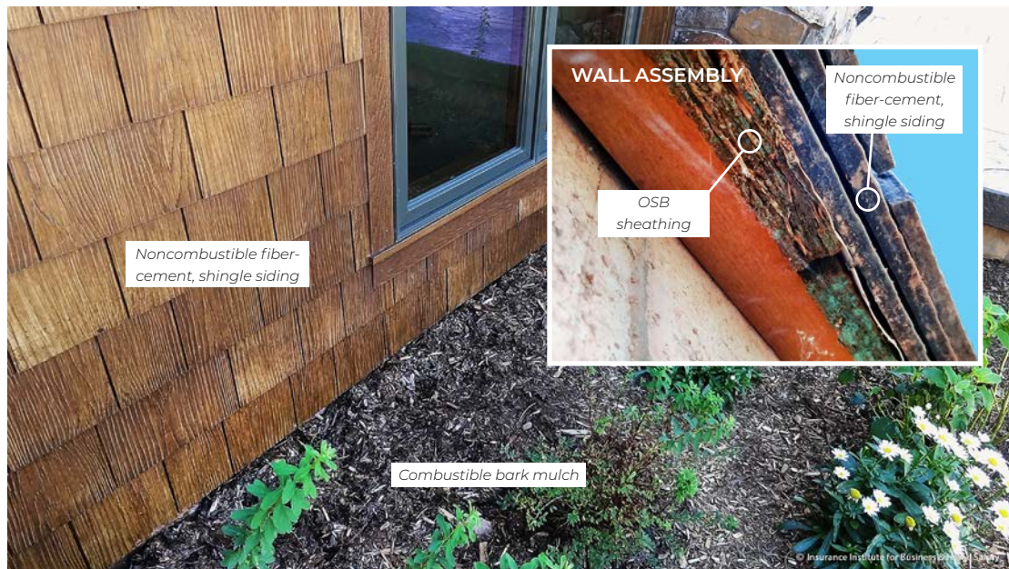
Figure 20. Wall details show that even with noncombustible siding, combustible sheathing and wall framing can be exposed. Without the 6-in. vertical noncombustible zone, the sheathing and framing are susceptible to ember accumulation or may be in contact with combustible fuels at the base of the wall.
